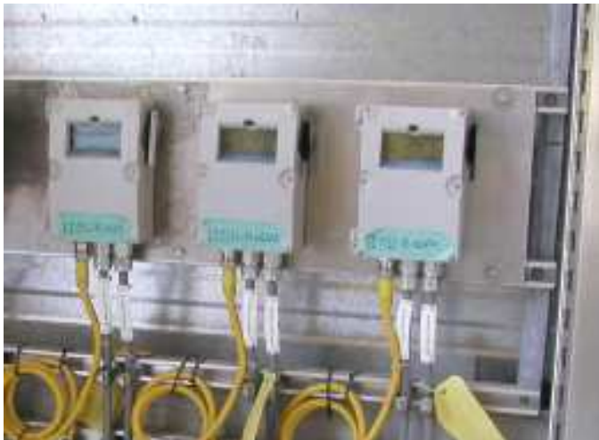
Figure 3 – Three of the units used in the installation: Milltronics MFA4p and Milltronics MSP-12 from Siemens.
