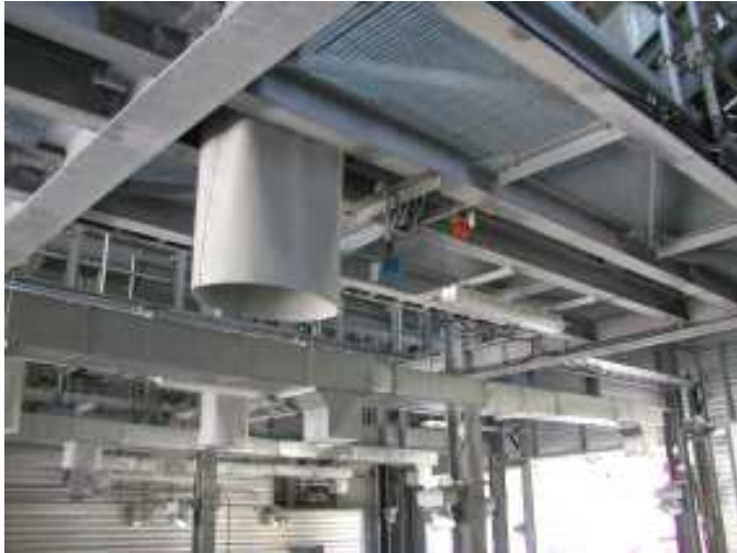
Figure 2 – An ultrasonic used to monitor sludge truck filling at the plant.
