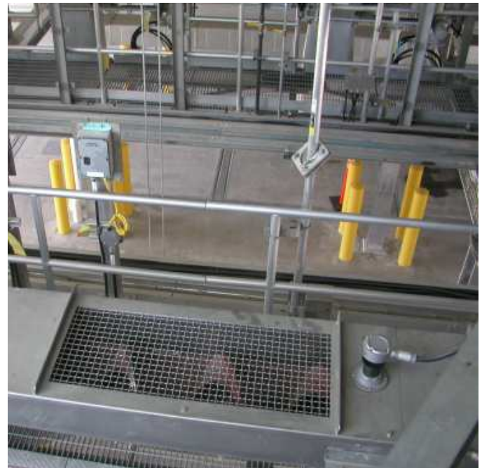
Figure 1 – A motion failure alarm controller provides reliable alarming directly to the Seymour-Capilano Filtration Plant’s control room.
