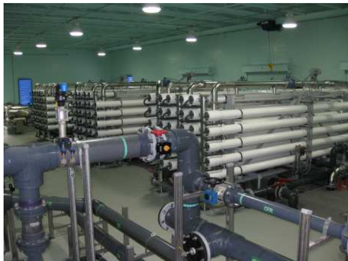
Figure 2 – Photo of a typical RO filtration installation
