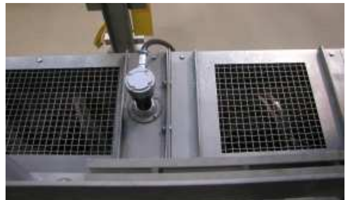
Figure 2 – A motion failure alarm controller provides reliable alarming directly to the Seymour-Capilano Filtration Plant’s control room.
