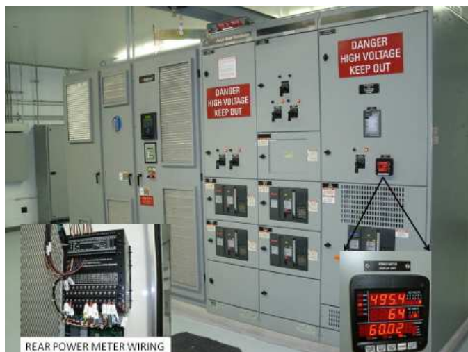
Figure 6 – Power Monitoring Equipment at MCC
